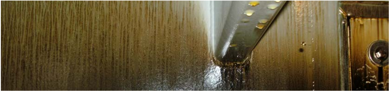
Varnish formation inside a GE 7FA turbine reservoir
